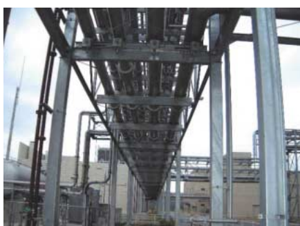
Example of overhead piping
