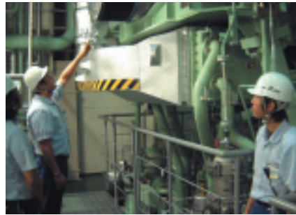
Gas engine in the cogeneration system
