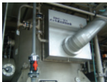
Evaporator of concentrator for alkaline and acid waste liquids
